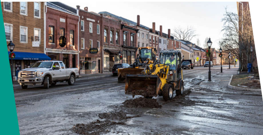
Cleanup of silt from the flood on Water Street in Hallowell, Maine. PHOTO BY DAVE DOSTIE
