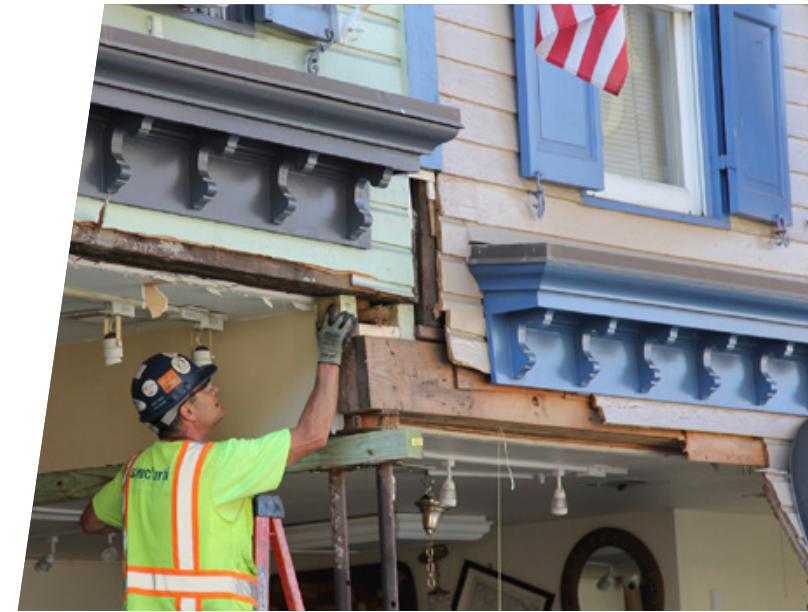
Building stabilization after severe flood damage in Ellicott City, Maryland. PHOTO BY PRESERVATION MARYLAND
